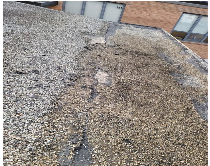
Before # 2 Split in Membrane needs to be repaired.
