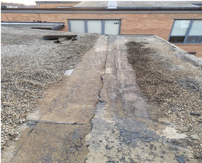
Before # 1 Split in membrane needs to be repaired.
